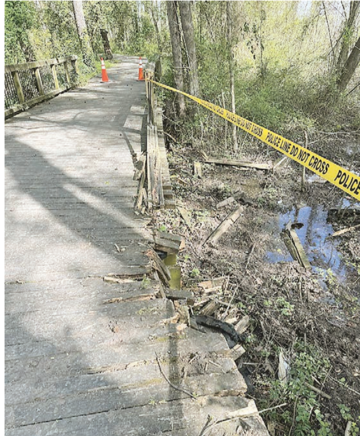
Car left the parkway and hit bike trail bridge #21.
